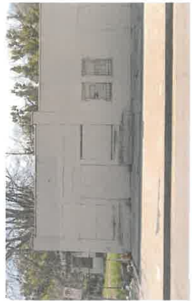
Uninhabitable Commercial Property Source: Google Street View
