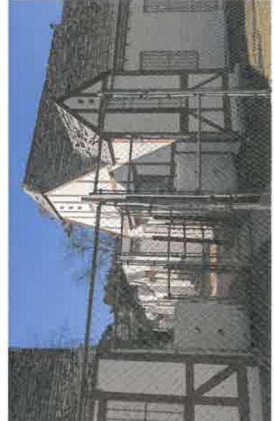
Uninhabitable (as determined by interior inspection) Multifamily Homes Source: Given Associates
